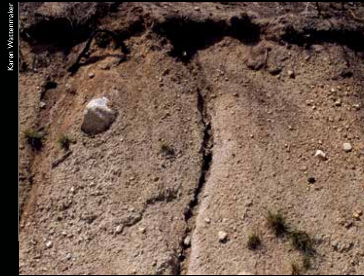
Erosion – Surface erosion.
