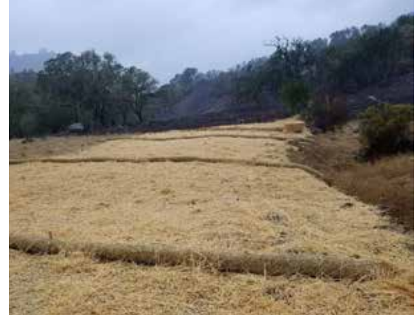
Loose straw mulch and straw wattles are among the methods used to prevent soil erosion and debris runoff at Kimball Reservoir following the Tubbs Fire. Photo from Calistoga Public Works Staff
